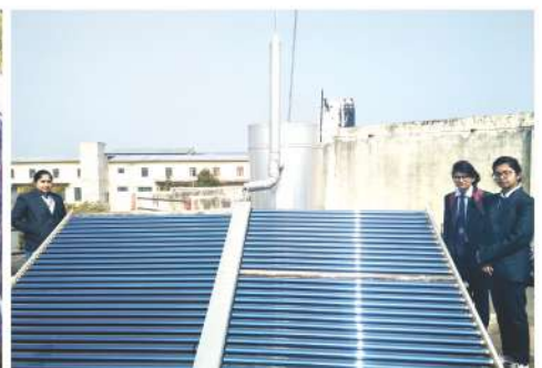
Solar power water heating plant (EE)
